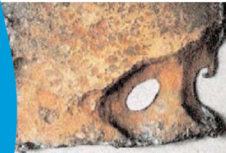
The above is typical sulphate reducing bacteria corrosion pitting of a diesel oil storage tank 10 mm bottom plate, which occurred within nine months.
